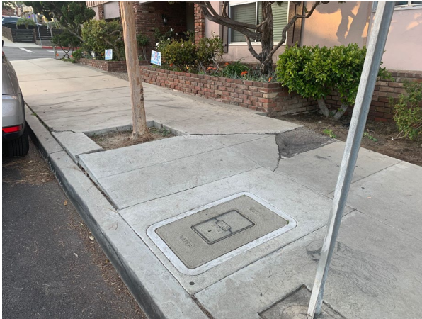
Before: 1003 E. Pine uplifted sidewalk
